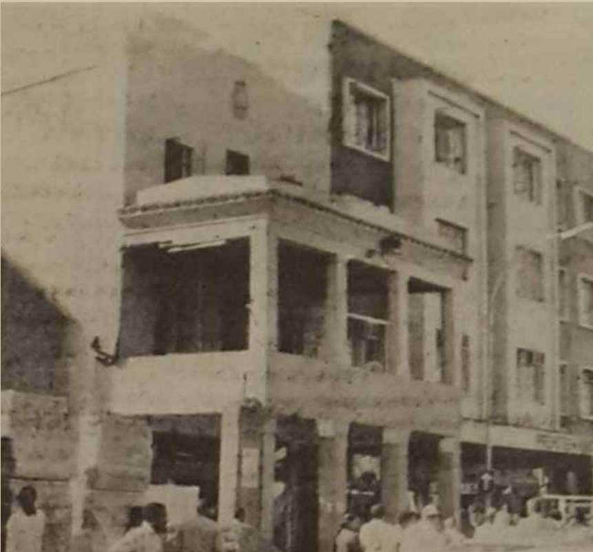
The building which has been vacated because of sagging foundation.
