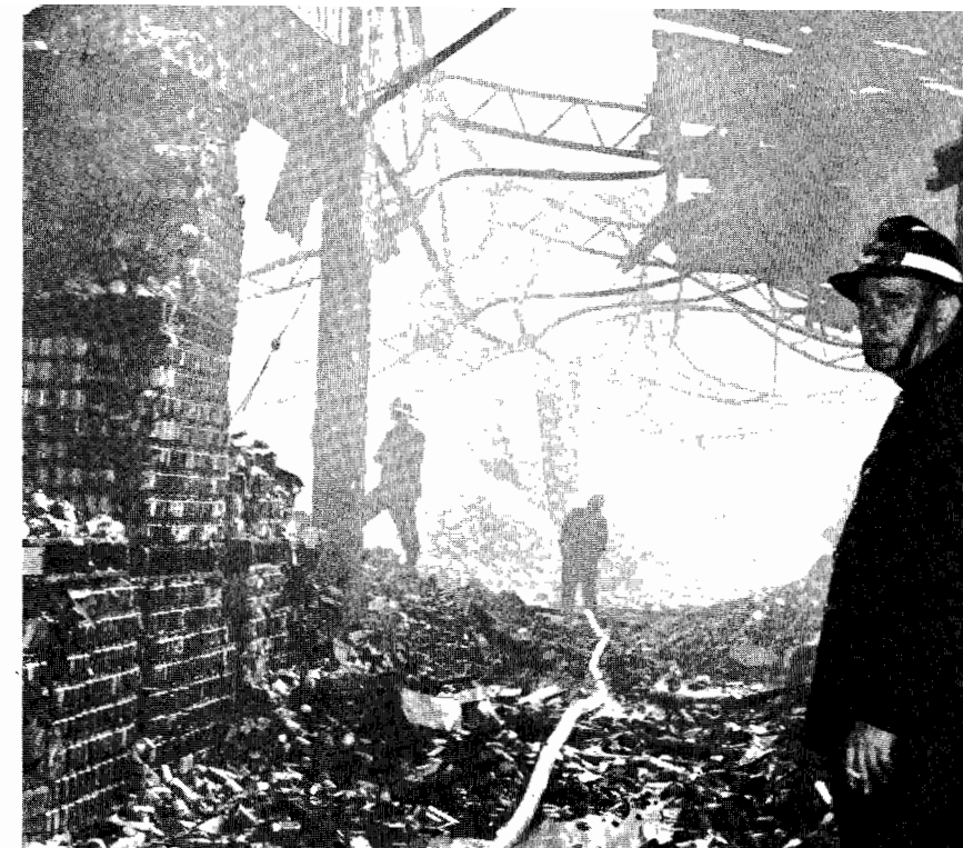
A beautiful home gutted by fire.
